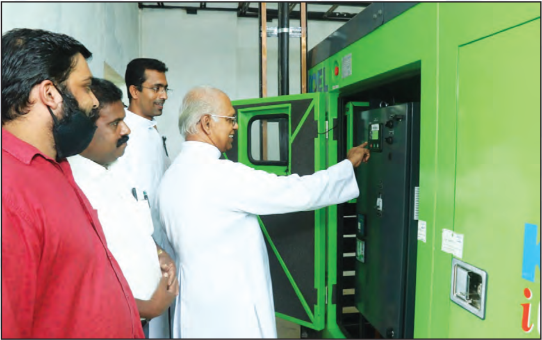
Inauguration of High Tension Electricity Supply Unit
